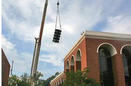
A crane lifts one of the sirens for LaGrange College’s outdoor warning system onto the roof of Henry Hall.
